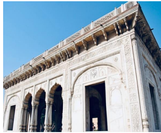
Figure 14: The carved brackets support the intricate jali work on the parapet wall.
